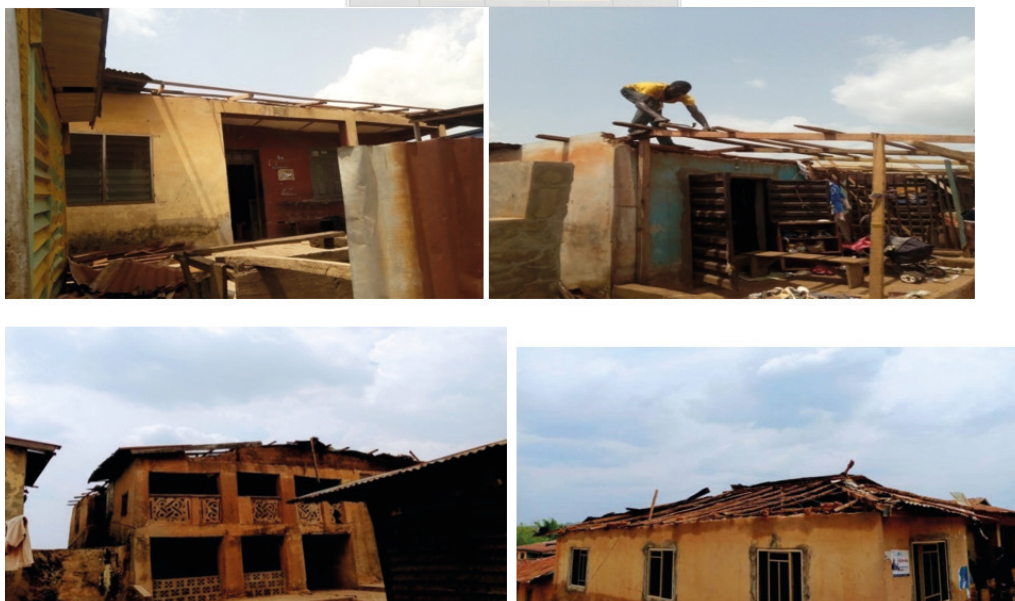
Figure 1. Some of the buildings were affected by the rainstorm of 3rd March 2023 in the study area.
