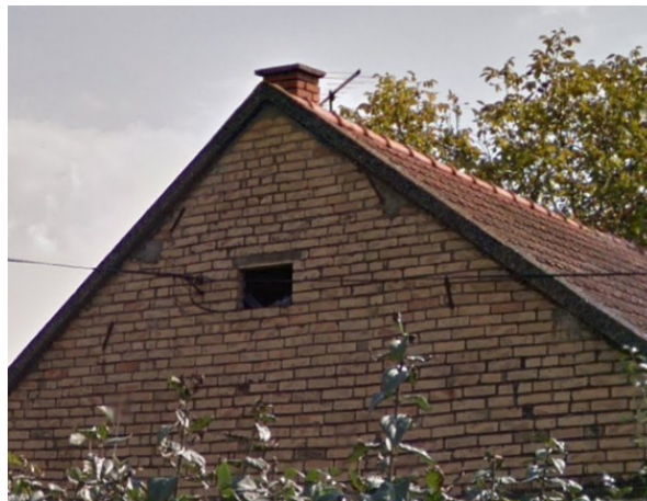
Figure 14. One brick row without reinforcement, with little open windows for ventilation. The wind can enter through this window and lift a few roof tiles, opening the space for more to blow off. In the case of a one-brick row without internal reinforcement, it can be demolished by a high wind gust. Google Street Imagery 2014.
