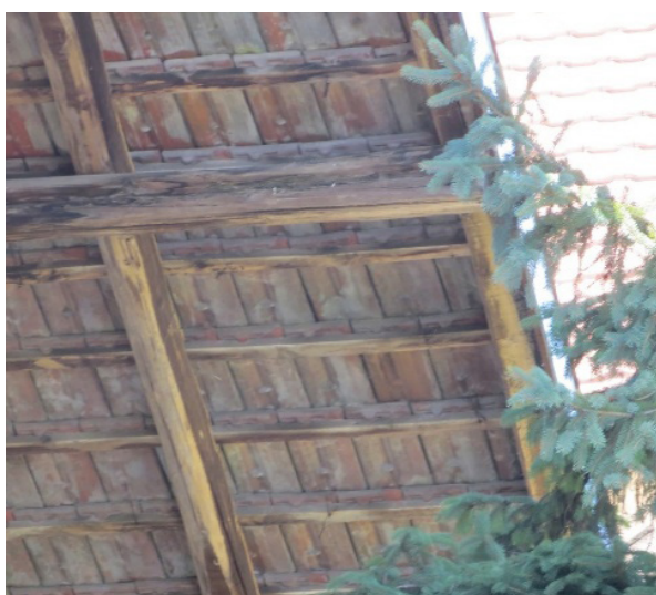
Figure 8. Non-closed roof with closed doors and windows on the non-roof sides. During the windstorm, all roof tiles will be uplifted on this exposed roof construction example.
