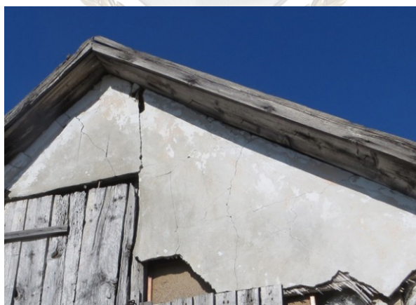
Figure 15. Wooden door, reed, and plaster without reinforcement.
