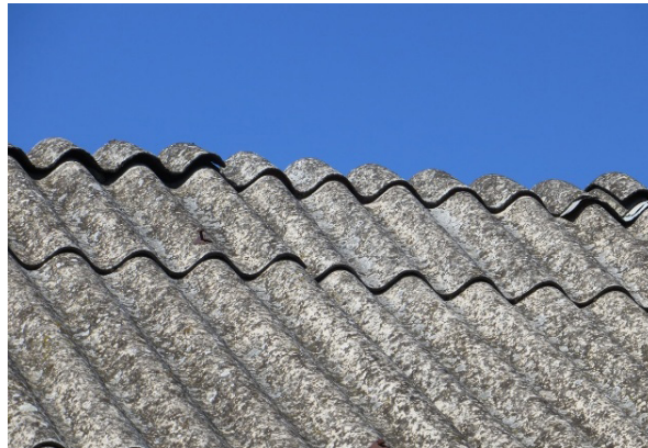
Figure 16. Asbestos roof sheets. This type of roof material is highly vulnerable because it is fragile and can be lifted in one piece during windstorms.
