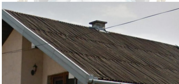
Figure 18. Bitumen roof sheets. This example shows the highly vulnerable roof with irregular bitumen roof sheets damaged by the sun. Google Street Imagery 2014.
