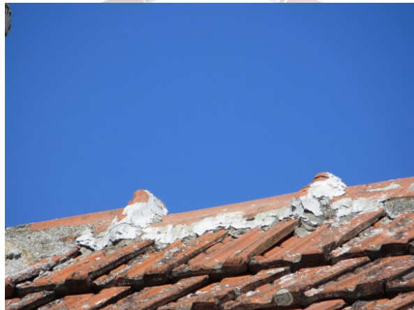
Figure 11. Roof ridges sealed with plaster. This step will prevent the blowing of roof ridges and expose the top of the roof to wind.
