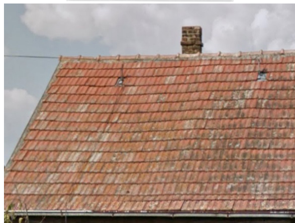
Figure 12. Roof tiles and ridges sealed with plaster. Google Street Imagery 2014.
