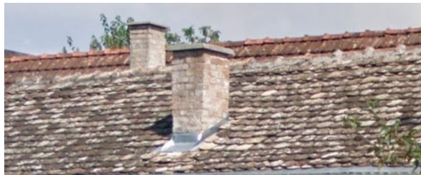
Figure 17. Biber plain roof tile. This type of roof material is highly vulnerable because it is fragile, lightweight, and can be easily lifted during windstorms. Google Street Imagery 2014.
