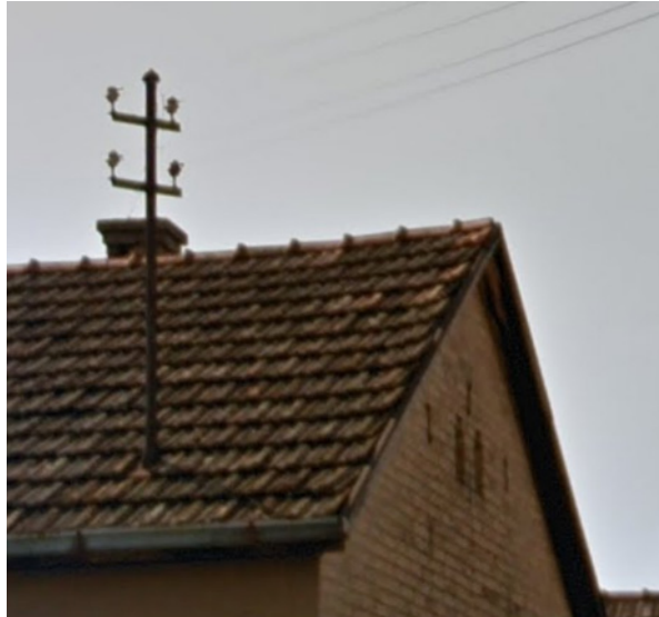
Figure 10. Roof ridges and roof tiles on the edges of the roof are not sealed, and there are no metal rakes on the edge of the roof. During the windstorm, the first row of roof tiles will be uplifted, creating more space for wind to enter beneath the tiles and blow them away. Google Street Imagery 2014.
