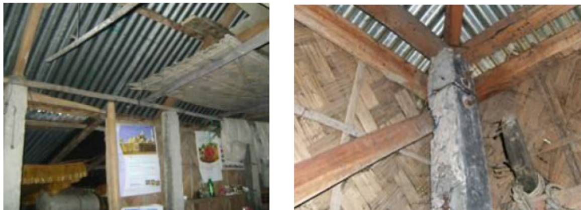
Figure 19. A Loose connection of timber with R.C.C. pillar makes the structure vulnerable, and using nuts and bolts frequently makes the post less intense. (Source: Shelter Cluster).
