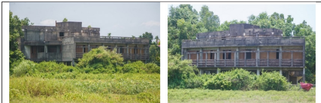
Figure 17a. Existing condition of DASCOH Cyclone Shelter (Photo: Author)
